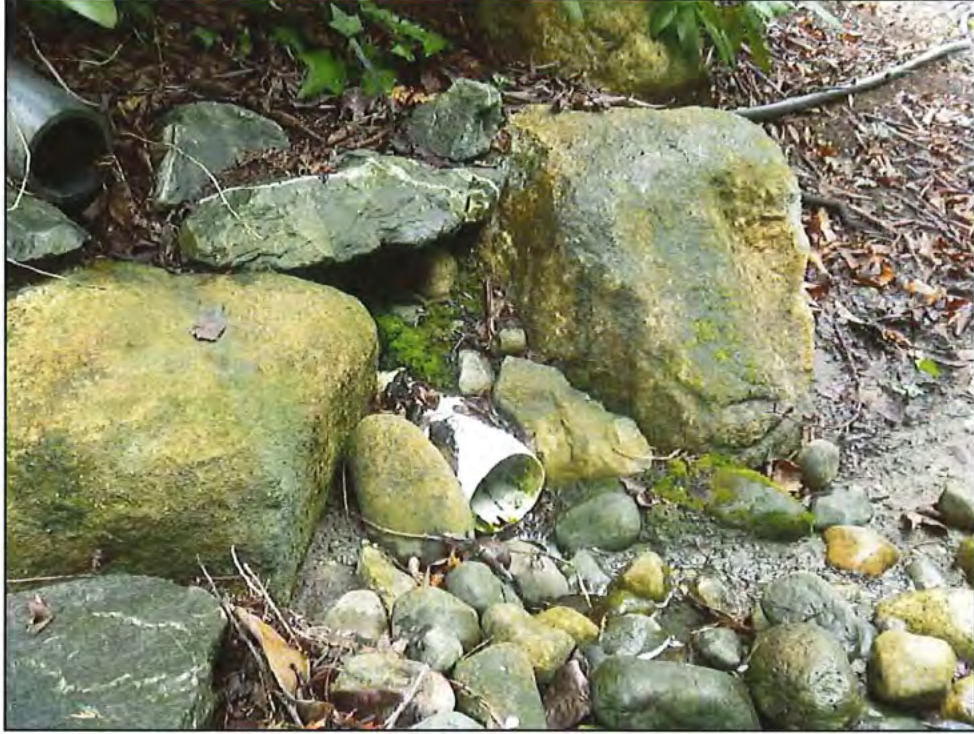
Photo 3. One of the observed drain pipes from adjacent homes.
